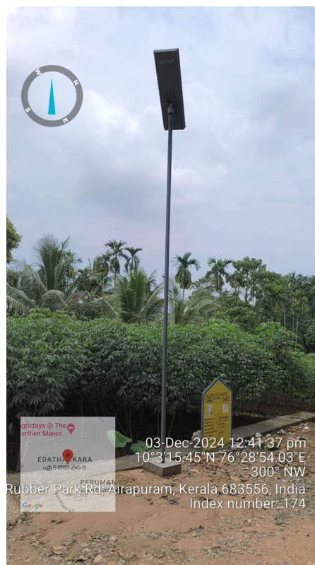
Solar Street lights
