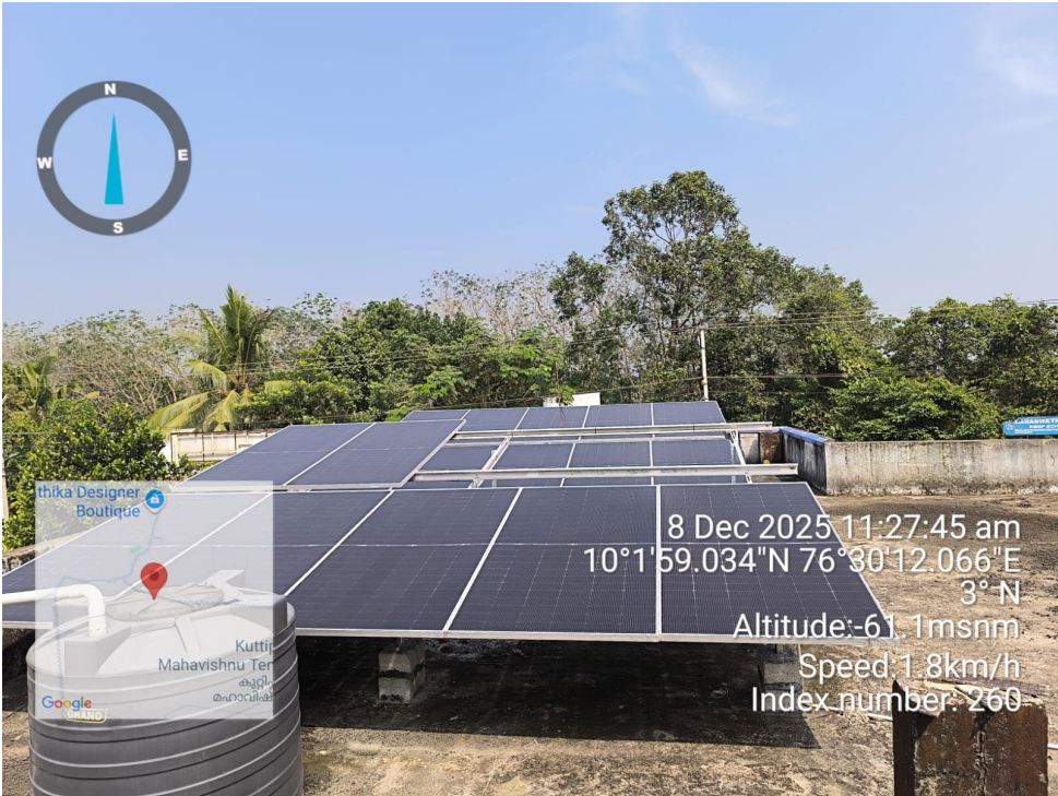
Solar panel installed at the project
