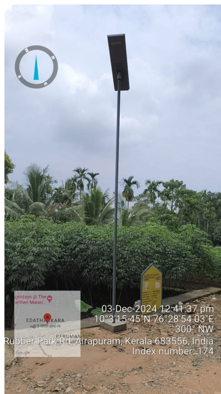
Solar Street lights
