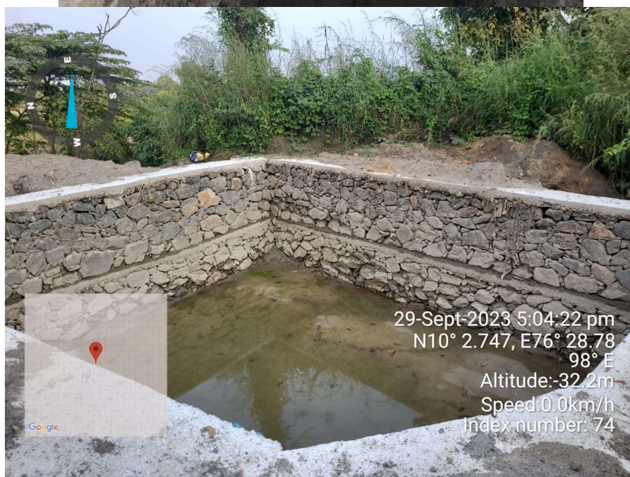
Drainges and siltation trap
